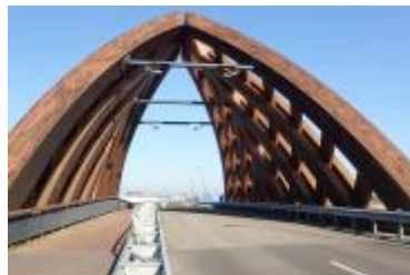
Figure 12: bridge with degraded paint layer.
