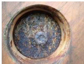
Figure 3: Bridge and its metals components. Behind a removed wooden plug water accumulated appeared causing corrosion on the metal parts.
