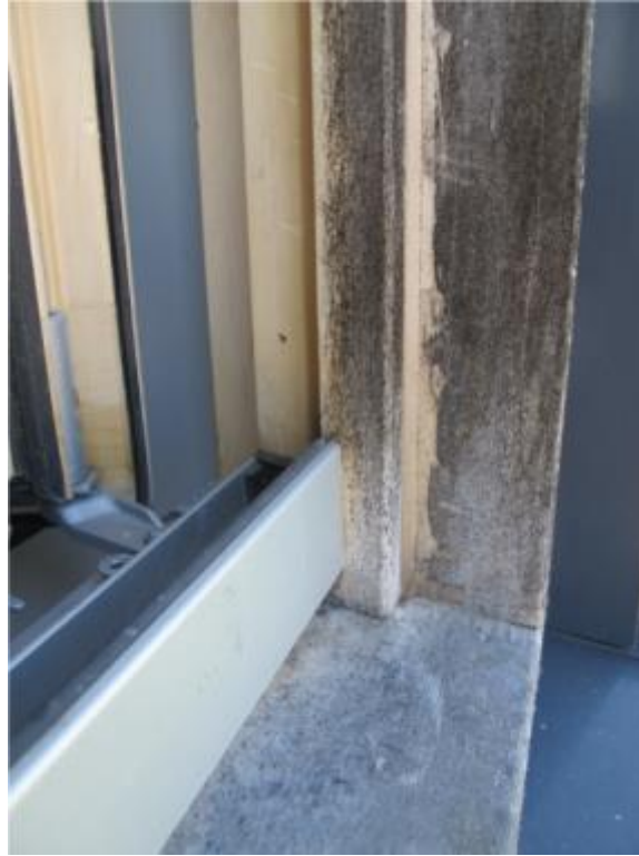
Figure 15: differences in discolorations and mould growth.
