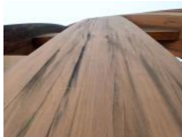
Figure 9: postcentral column with cracks.
