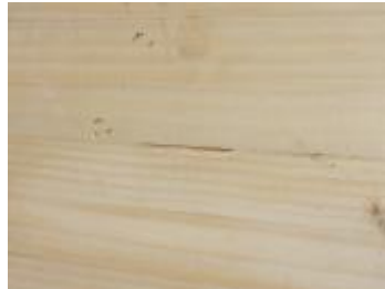
Figure 8: Beam in cycle track Assen with a removed shallow peel which was a result of a drying crack.
