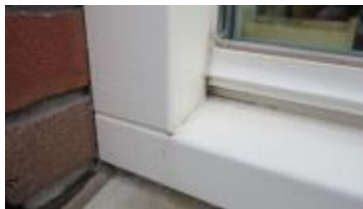
Figure 6: Joinery with small humps near the corner.
