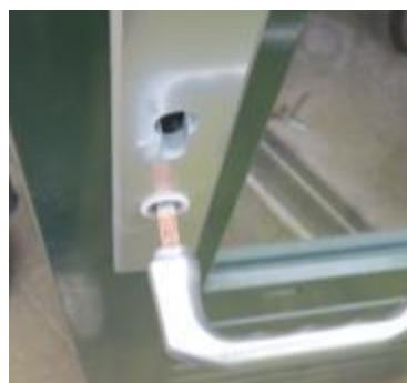
Figure 4: Sheet door which stood frequently open causing water accumulation in the lock resulting in corrosion on the metal parts.
