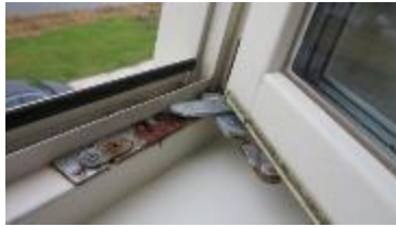
Figure: 5 Window with high and long term condensation causing corrosion on the metal parts.
