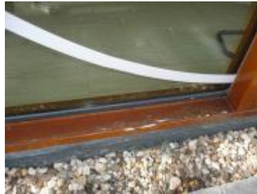
Figure 11: Window frame with high moisture content causing paint damage.
